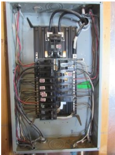
Electrical Electrical Panel
