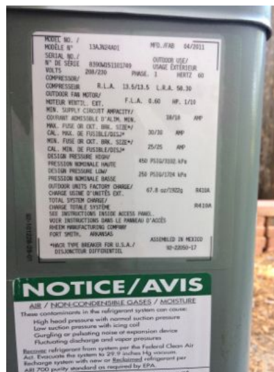
Heat/AC AC Compress Condition
